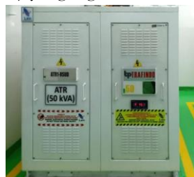
Gambar 4. Auxiliary Transformator (ATR)
